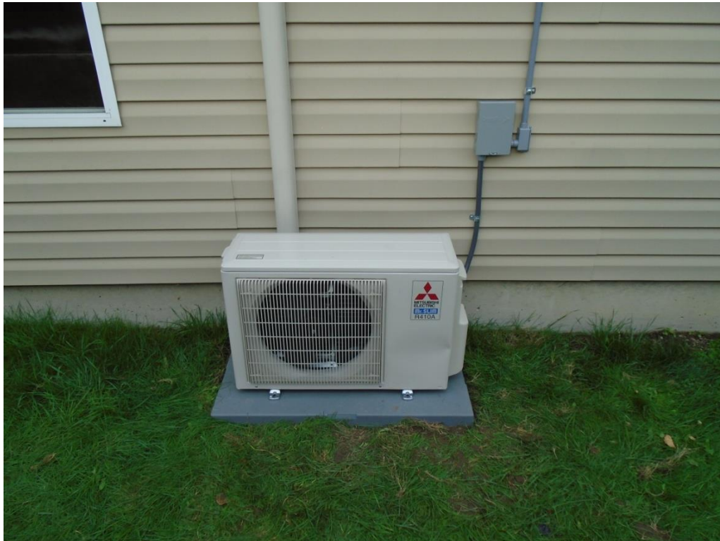
Figure 2. DHP Outdoor Unit – Tacoma WA
